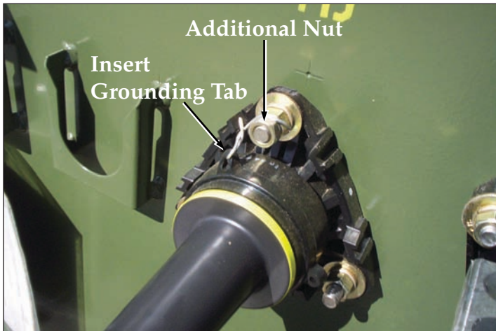
Figure 3 Option 2 – Bushing Well Insert with a #14 ground wire wrapped around stud with nut added.
